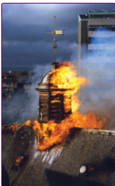
Fire severely damaged the Bower Building, University of Glasgow.
