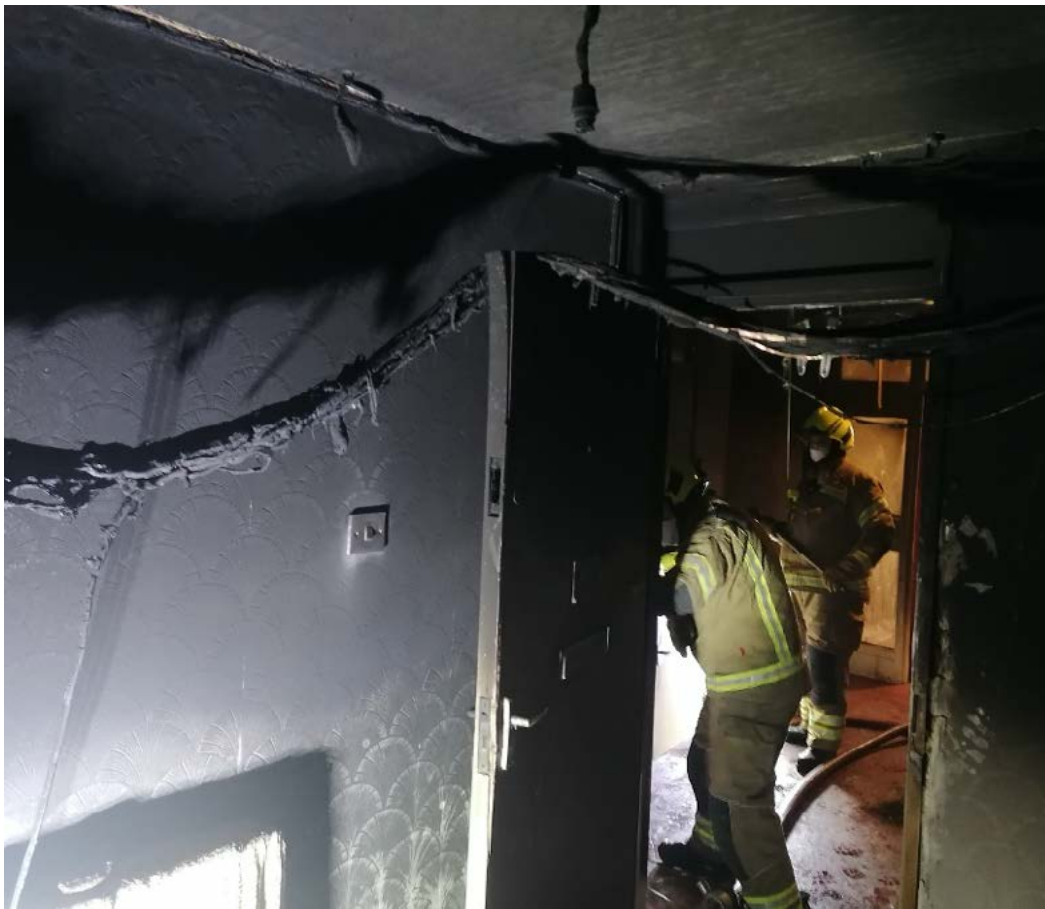
Figure 7: Dislodged cabling Source: SFRS
